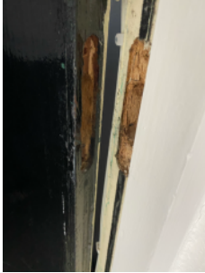
PERKO self closing device has been removed - F.E.D flat 7
