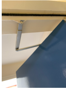
A working self closing device fitted on entrance door to flat 7.
