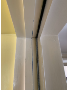
Intumescent strips and cold smoke seals on entrance door to flat 7.
