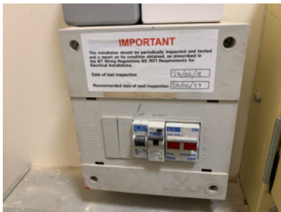
Electrical installation with current test label.
