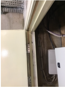
Missing strips and seals
