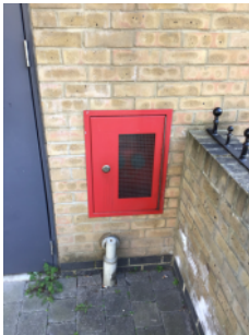
Dry riser inlet
