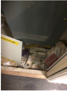
Combustibles in ground floor electrical cupboard
