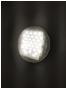
Maintained EL within the staircase
