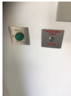
Electromagnetic door release with emergency backup at main entrance door
