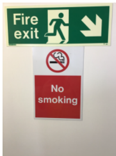
Escape route signage
