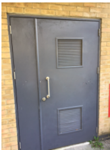
External secure bin store
