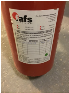
Extinguisher test date of 2012
