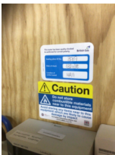
Evidence of gas meter inspection
