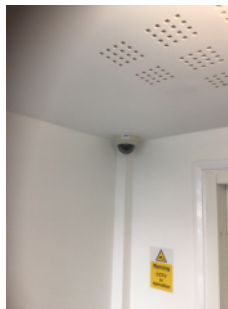
CCTV cameras are provided
