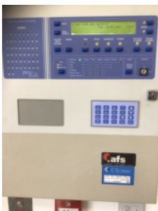
Main fire alarm panel
