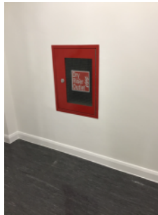
Dry riser outlet on each landing
