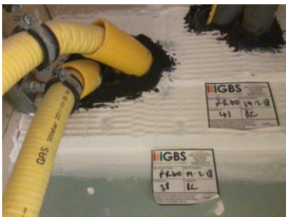
Evidence of fire stopping within riser cupboards conducted in 2018
