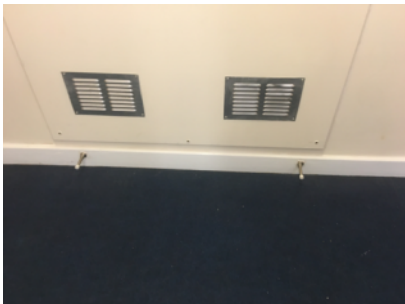
Confirm grill-vents are intumescent protected
