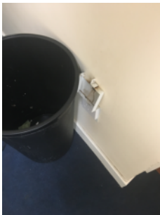
Electrical sockets in common area with lockable covers
