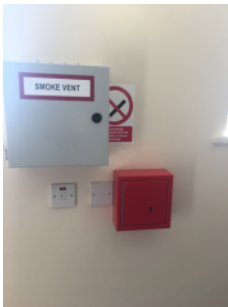
Smoke vent control panel.
