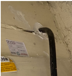
Fire stopping within electrical cupboard.
