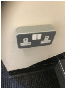
Electrical sockets in staircase
