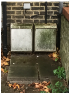
Gas meters located externally
