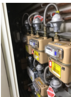
Gas meters in riser cupboard
