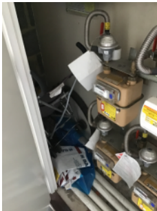
A pram, and other combustibles in the gas meter cupboard, ground floor.
