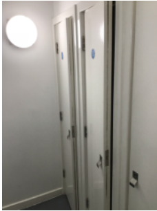
Unlocked riser cupboards
