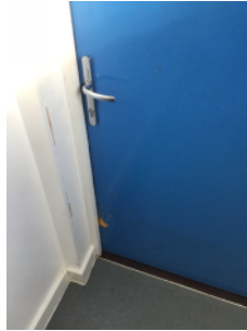
Damaged flat door
