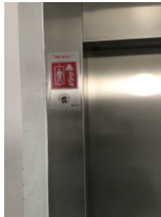
Firefighter override facility
