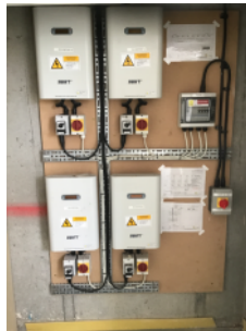
Electrical Inverters from wind turbines located on the roof.
