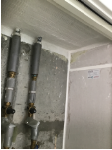
Example of fire stopping within risers
