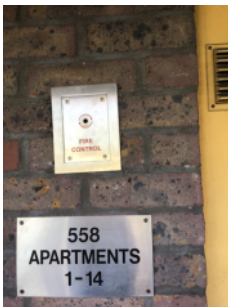
Firefighter override facility
