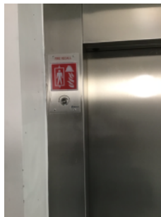
Firefighter override facility
