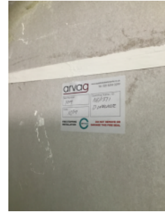
A programme of fire stopping within riser cupboards was carried out in 2019
