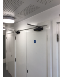
Ground floor riser cupboards
