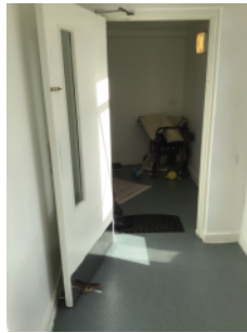
Combustible storage in a third floor lobby outside flat 12
