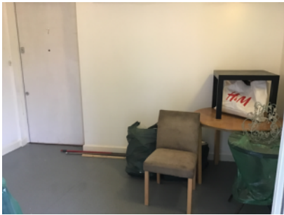
Combustible storage on second floor outside flat 7
