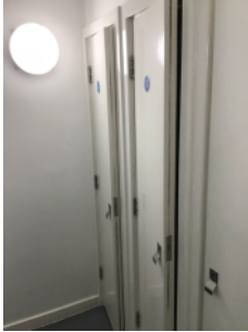
Unlocked riser cupboards
