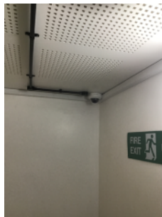
CCTV provides on the ground floor.
