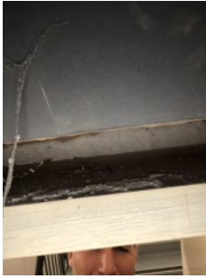
Fire stopping required around door frames inside riser cupboards
