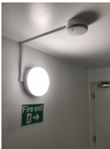
Signage pointing wrong direction
