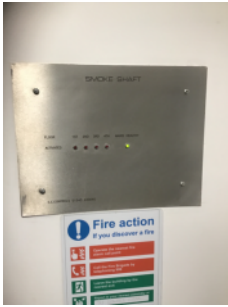
Smoke Shaft showing in “healthy” condition
