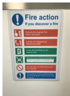
Incorrect Fire Action Notice should be removed
