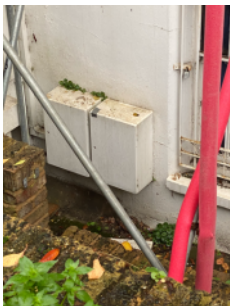
Gas meters located externally
