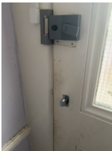
The provision of a thumb turn device on the final exit.
