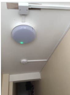
Emergency light within common hallway
