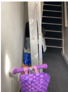
Items obstructing escape route
