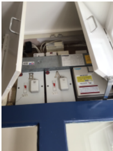
Small ceiling level electrical cupboard
