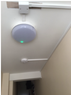
Part 6 system in hallway
