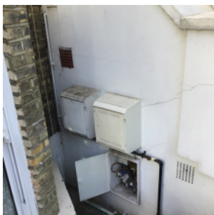
External gas meter cabinets
