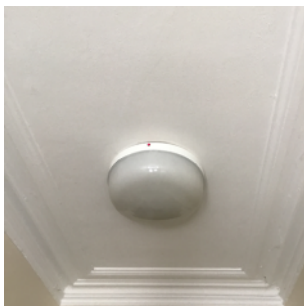
Red led light on emergency lighting unit
