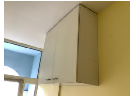
Electrical cupboard is not FR.
