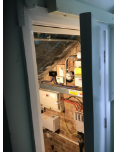
Electrical cupboard door, to FD30S standard.
