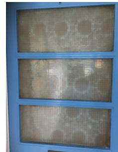
Georgian wired vision panels fitted in FEDs
