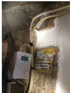
Fire stopping certification label, fire stopping in electrical cupboard.
