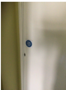
“Keep Locked Shut” signage on the electrical cupboard door.
