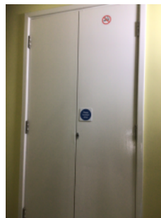
“Keep Locked Shut” signage on riser doors.
