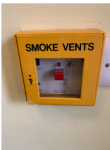
Manual Smoke Vent Control
