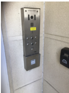
Fob access to the main entrance door
