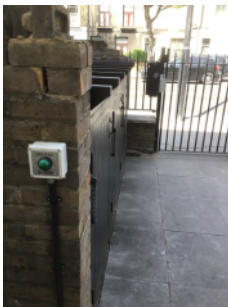
Electromagnetic release device for the main gate.
