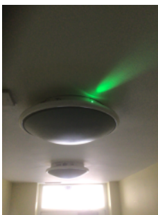
Maintained EL is provided within the staircase.
