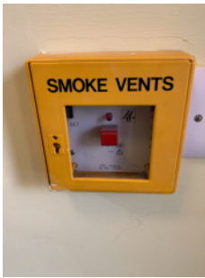
Manual Smoke Vent Control
