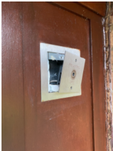
Defective entrance door override
