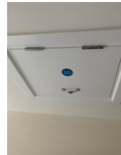
It was not possible to access the roof space within the scope of this FRA
