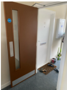
Lobby doors should not be wedged open
