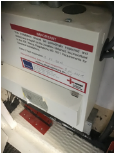
Electrical installations inspected May 2016
