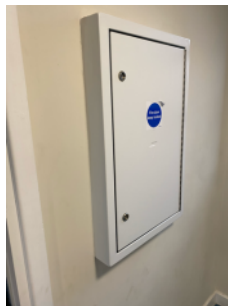
Electrical meter cupboards in common areas.
