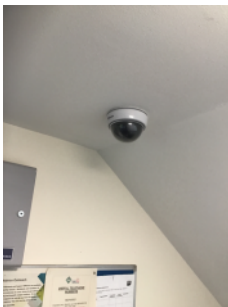
CCTV is provided
