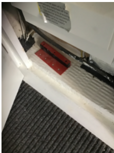
Fire stopping within electrical meter cupboards.
