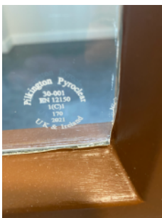
Acid etching on FR Glazing installed in lobby doors
