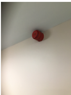
Fire Alarm Sounders provided within common parts.
