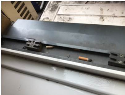
Evidence of smoking, staircase window, 1st floor
