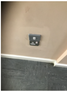
Electrical sockets in common parts
