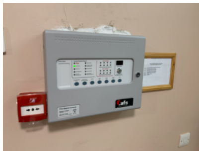
Fire alarm panel, with manual call point
