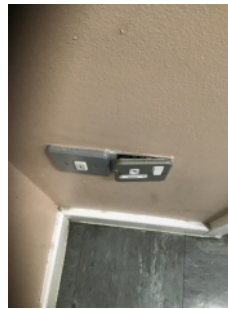
Electrical socket between the ground and first floor requires repair
