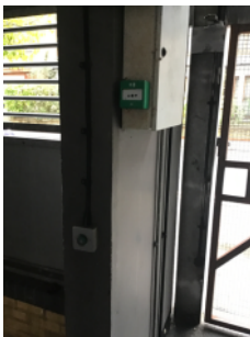
Defective rear gate electromagnetic release and emergency release.
