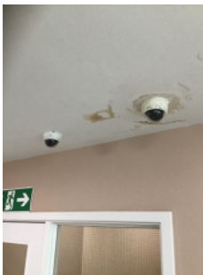
CCTV is provided
