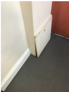
Example of boxed in services in the building, affording no fire resistance
