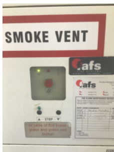
Smoke vent panel - with no evidence of maintenance since 2019
