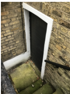
It was not possible to access this door
