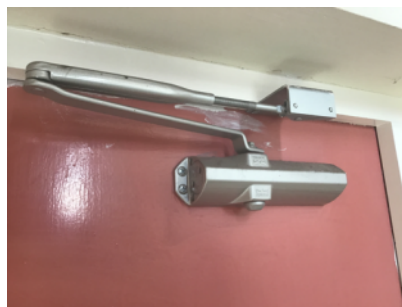
Example of externally fitted self closing device fitted to all flat doors
