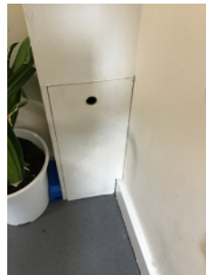
Example of boxed in services in the building, affording no fire resistance
