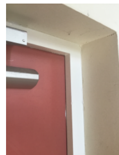
Example of door stops on all flat entrance doors.
