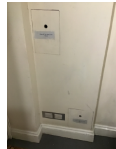
Example of boxed in services in the building, affording no fire resistance
