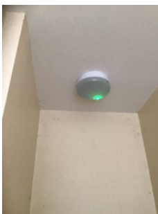
Maintained emergency light (local) provided in entrance hallway.
