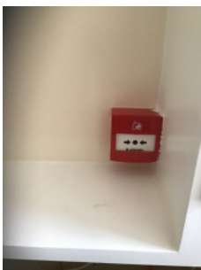
Manual call point provided in common hallway.
