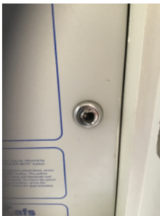
Damage to panel keyhole
