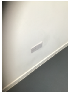
Electrical sockets are provided in common areas on all floors.
