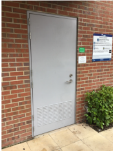
Access could not be gained into the gas room located externally
