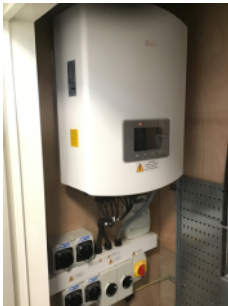
Three Phase Inverter located in the electrical riser cupboard.
