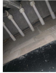
Pipe penetrations, without fire stopping, in the gas and water riser
