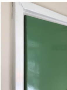
Lobby door not closing fully
