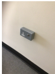
Electrical sockets are provided in the common staircase
