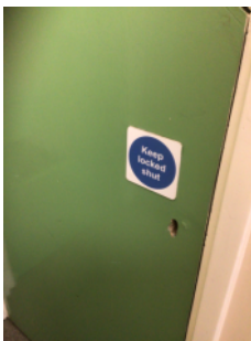
Fire door signage on locked fire doors
