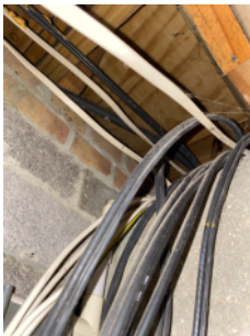
Cable penetrations in the second floor riser cupboard
