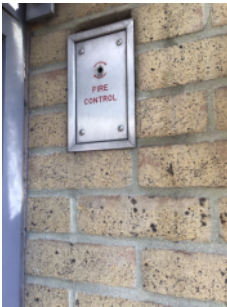
Defective override facility
