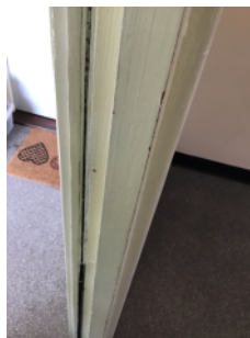
Missing section of smoke seal
