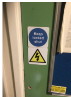
Fire door signage on locked fire doors
