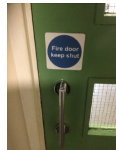
Fire door signage on self-closing fire doors
