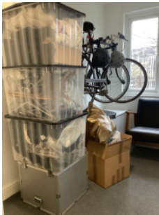
Combustibles and obstructions on the staircase
