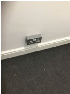
Electrical sockets provided in common staircase
