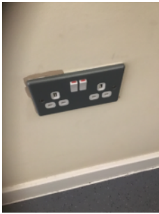
Electrical sockets in communal staircase
