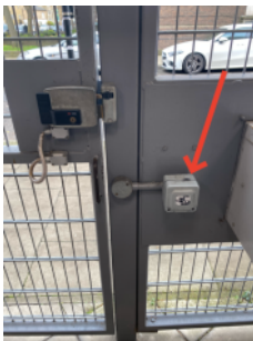
Release switch for gate is located in this box
