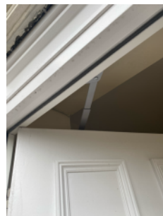
Overhead self closing device, Flat 33, observed to operate effectively
