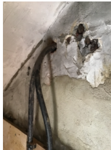
Cable penetrations without fire stopping in electrical cupboard
