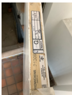
Certification label on electrical cupboard door
