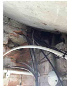
Lack of fire stopping in electrical cupboard
