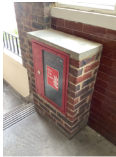
Dry rising main outlet on common balconies
