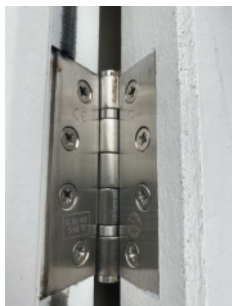
BS EN1935 fire rated door hinges on Flat entrance door, flat 33
