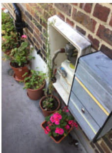
Example of Gas meter boxes with damaged/missing doors
