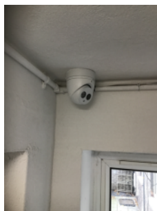
CCTV is provided internally
