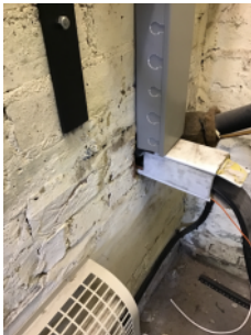
Cable penetrations without fire stopping in lift machine room
