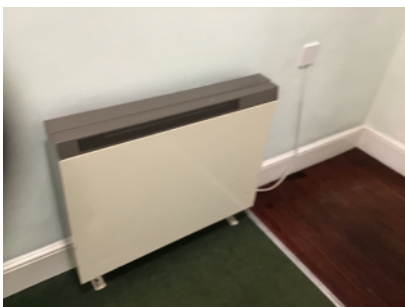
Storage heaters used in common areas
