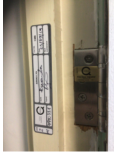
Certification of recently installed FR doors in riser cupboards
