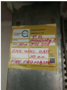
Fire stopping certification label in the electrical intake cupboard.
