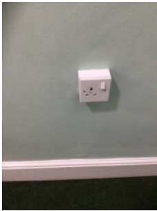
Electrical sockets provided in common areas.
