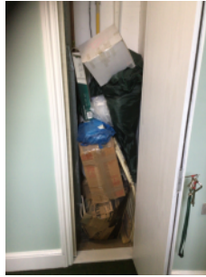
Example of high volume of combustibles in riser cupboards
