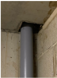
Soil pipe penetration without fire stopping within the bin store.
