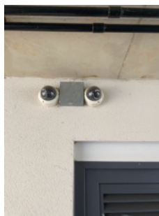
CCTV cameras are provided
