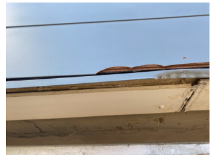
A damaged area exposes the core of the laminate EWS on front elevation.
