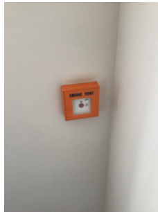
Smoke vent manual override switch.
