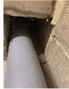
Soil pipe penetration without fire stopping within the bin store.
