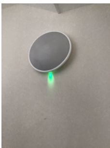
Emergency lighting in staircase
