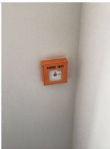
Smoke vent override
