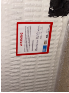
Fire stopping certificating label in riser cupboards.
