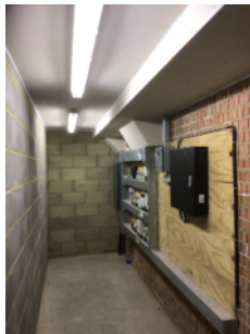
Good standard of compartmentation within the 1st floor electrical cupboard
