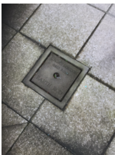
Lightning system earth rod.
