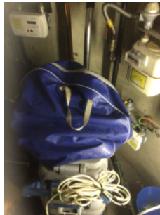
Heavy cleaning machinery located against gas installations.
