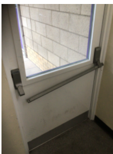
The panic exit device requires urgent repair.
