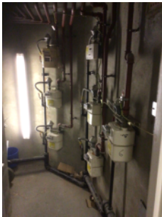
Gas meters located in a bespoke cupboard.
