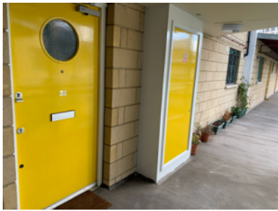
Showing glazed fanlights in doors and glazed flat windows (all above 1.1m)
