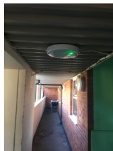
Maintained emergency lighting provided on common balconies
