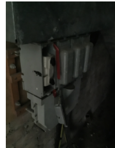
Damaged fuse box
