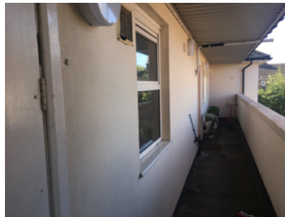
Photograph showing vents & glazed windows above 1.1m on common balconies
