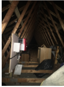
Roof space without fire separation.
