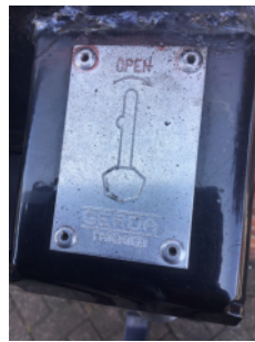
Fire service entrance gate override function.
