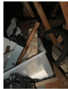
Combustible storage in the roof space
