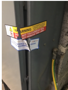
Broken seal in electrical cupboard
