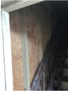
Plywood staircase separation.
