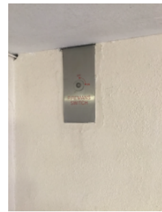
Lift fireman's switch
