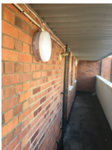
Maintained emergency lighting provided on common balconies
