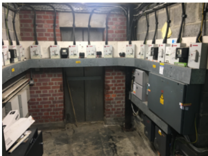
Electrical installations in electrical cupboard
