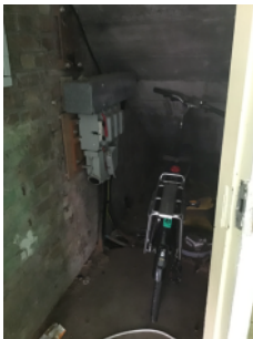
Bicycle in electrical cupboard
