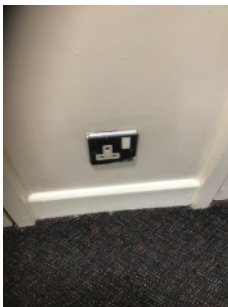
Electrical socket in common staircase
