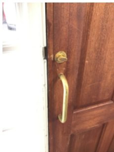
Thumb-turn device on main entrance door.
