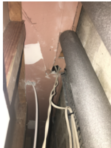
Example of pipe and cable penetrations in riser cupboards.
