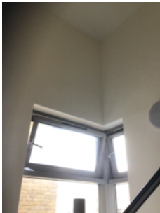
Uppermost staircase window at a height lower than uppermost staircase door
