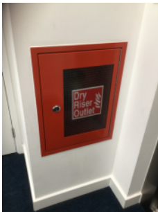
Dry riser outlet provided on each floor within the staircase
