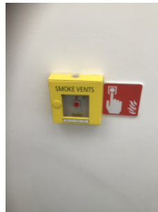
AOV in staircase is provided with additional manual smoke vent actuators
