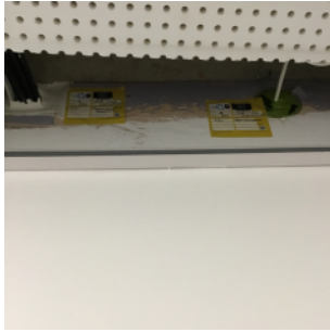
Version 4 - 17/11/21 evidence of fire stopping above flat 15
