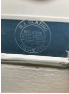
“Pyroguard” acid etching on staircase door glazing and glazed panel
