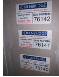
Example of fire stopping certification labels in risers
