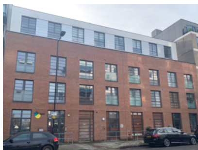
Front elevation, with unidentified external wall system on 3rd floor.
