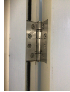
Door hinges to BS1935 and CE1121 on FD30S staircase doors
