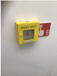
Smoke vent actuator for head of stairs clearly identified
