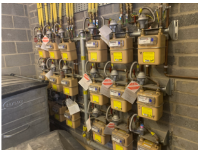
Gas meters located in bin store.
