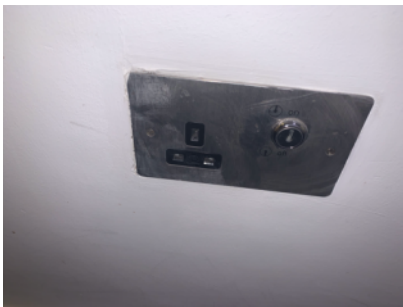
Key operated electrical sockets in common corridors
