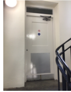
It was not possible to access this door: non standard lock fitted
