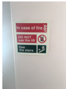
“Do Not Use Lift” signage provided
