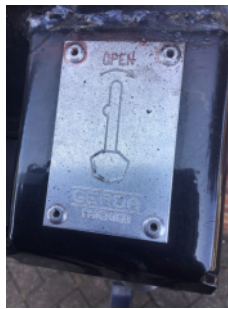
Fire service entrance gate override function.
