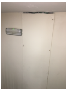
Non maintained lighting in the staircase
