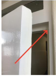
Lift lobby doors, no strips and seals, however 25mm door stops
