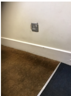
Electrical sockets in the common staircase
