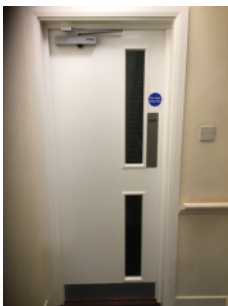
“Fire Door Keep Shut” signage on lobby doors
