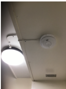
Example of the Part 6 alarm provided in common parts.
