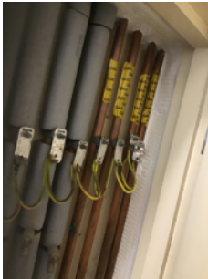
Fire stopping within the gas/water riser cupboard in entrance hallway.
