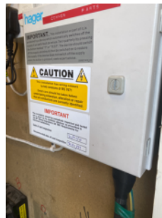
Electrical installation last tested in May 2018
