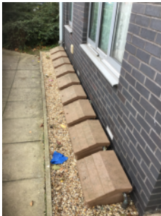
Gas meters located externally
