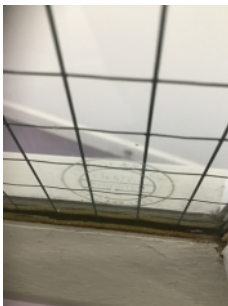
Acid etching on glazing installed in lobby doors.
