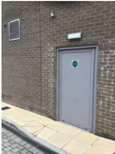
Access could not be gained here to assess standard of compartmentation
