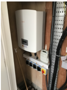
Three phase inverter, located in the 3rd floor electrical riser cupboard
