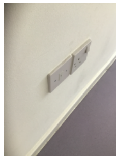
Electrical sockets are provided in common areas of the building
