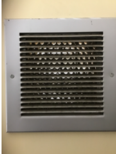
Vent grills fitted in riser doors appear to be intumescent
