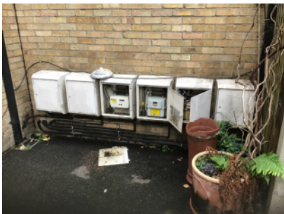
Gas meters are located externally.
