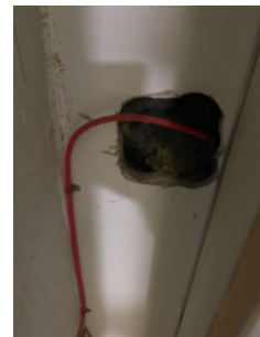
Cables penetrating from electrical riser cupboards into common parts.
