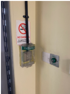
Electromagnetic door release, with additional emergency door release device
