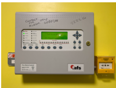
Fire Alarm control panel
