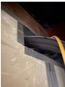
Cables penetrating from electrical riser cupboards into common parts.
