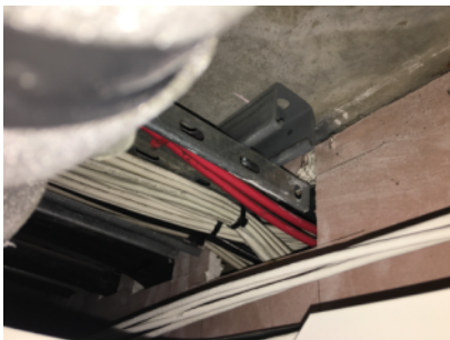
Cables penetrating from electrical riser cupboards into common parts.
