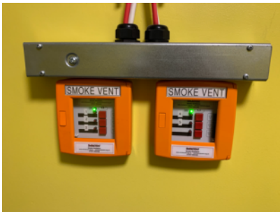
Smoke vent controls.
