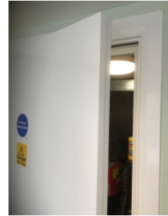
Electrical cupboard door to FD30S standard.
