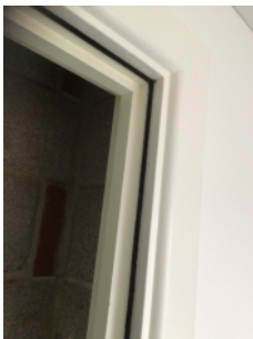
Intumescent strips and cold smoke seals have been fitted in riser cupboards
