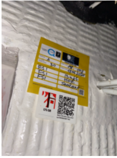
Evidence of fire stopping conducted throughout the building in June 2020
