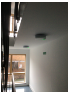
Maintained EL is provided in the staircase and within corridors.
