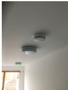
BS5839-6 smoke detection in the staircase
