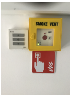
Smoke ventilation control
