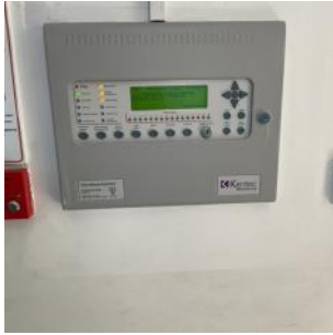
Fault lights on fire alarm panel
