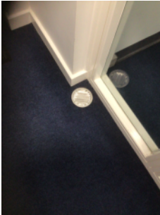
Gas vents in common corridors
