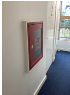
Dry riser main
