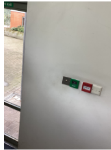
Exit devices and emergency override
