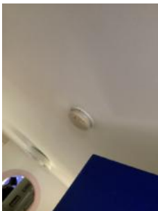
Flat 19 smoke alarm
