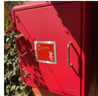
Premises Information Box
