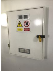
Non FR electrical cupboard on ground floor
