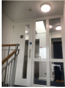
Partition compromising staircase AOV.
