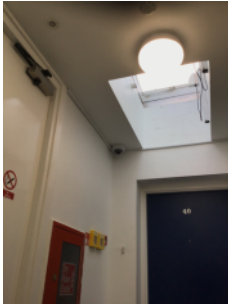
AOV located in 6th floor lobby.
