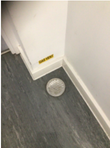
Gas vent in common corridors.
