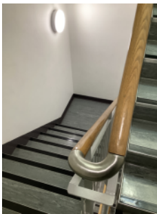
Escape route with contrasting stair nosings
