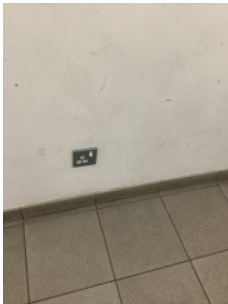
Electrical socket in common area
