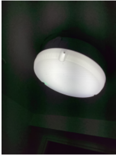
Emergency lighting unit
