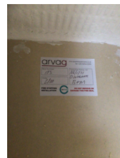
Fire stopping certification within riser cupboards
