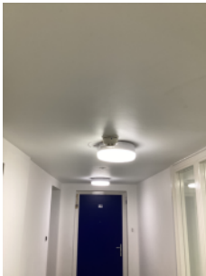
Smoke detector and sounder in common area
