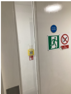
Escape route signage
