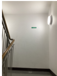
Inadequate escape route signage
