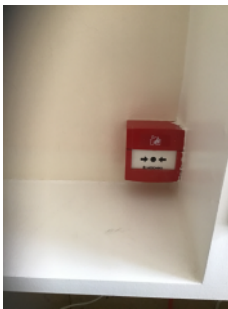
Manual call point provided in common hallway.
