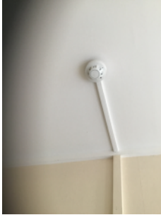
BS5839-1 detector located in entrance hallway.
