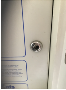
Damage to panel keyhole
