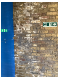
Escape route signage
