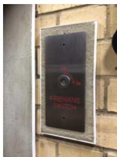
The provided lift is a fire-fighting lift.
