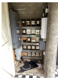
Electrical cupboard to the front of building
