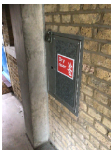
Dry riser outlets provided on each floor.
