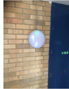
Maintained EL provided in the staircase.
