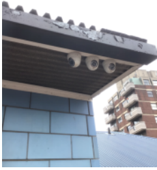
CCTV cameras are provided.
