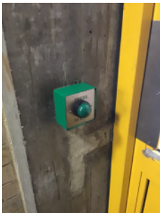
Exit device provided on main entrance door.
