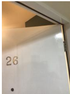
No self closing device fitted on flat 26 entrance door
