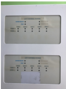
AOV control panel at ground floor
