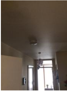
BS5839 Part 6 smoke alarm in Flat 8
