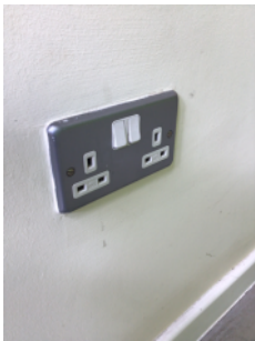
Double socket outlet in common area
