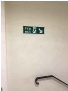
Escape route signage provided in staircase
