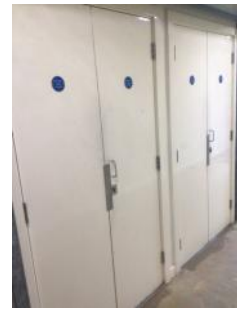
No access could be gained to ground floor cupboards
