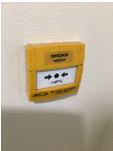
Smoke vent control
