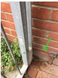
Lightning protection provided
