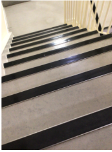
Colour contrasting nosing on stairs to aid with emergency evacuation
