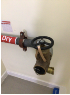
Dry riser outlet at head of staircase
