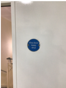
Appropriate keep shut signage displayed on lobby doors
