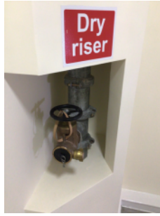
Dry riser outlet in staircase
