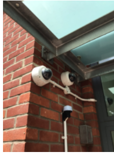
External CCTV coverage
