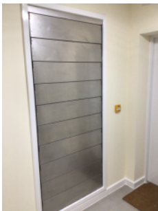
Smoke shaft in lobby
