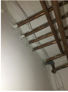
Example of fire stopping within riser cupboards.
