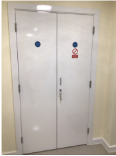
Riser cupboard doors found to be locked shut
