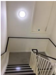
Stairwell normal lighting
