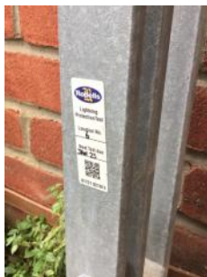
Lightning protection test label showing next test due in January 2025
