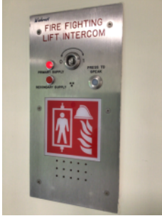
Fire fighting lift provided
