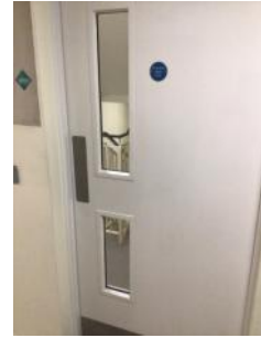
Fire resistant vision panel glazing to staircase / lobby door
