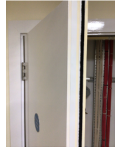
Doors to riser cupboards - FD60S standard
