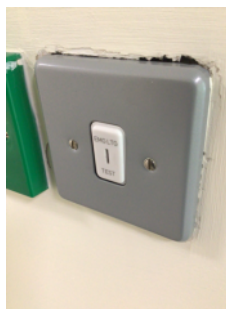
Emergency lighting test point
