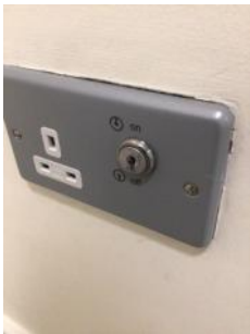
Key operated socket outlet in common area
