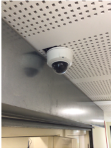
Internal CCTV coverage at ground floor
