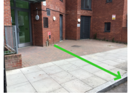
Dry riser inlet approximately 6m from kerbside
