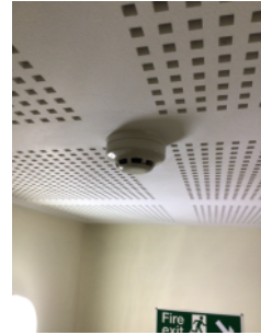
Part 1 detector at the head of the staircase to actuate AOV
