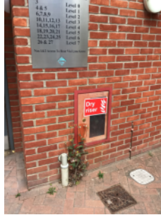
Dry riser inlet at main entrance to building
