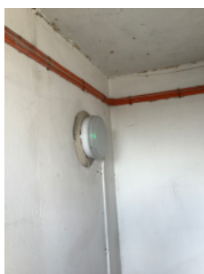
Maintained EL in the staircase
