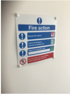
Incorrect fire action notice.
