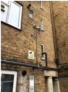
External CCTV cameras
