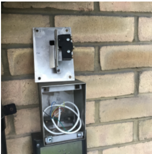
Defective Firefighter override facility
