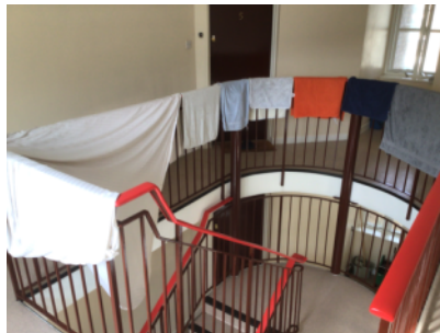
Combustibles located in common areas.
