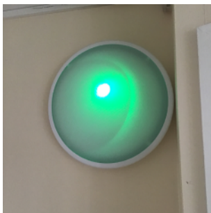
Emergency lighting in staircase
