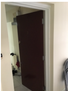
Flat entrance door with no self closer
