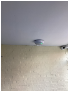
Emergency lighting unit in stairs
