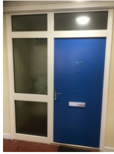
Recently fitted flat entrance doors, with FR Glazed panels & timber frames
