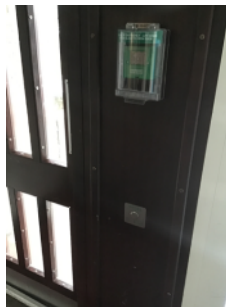
Main entrance door release, and break-glass emergency door release
