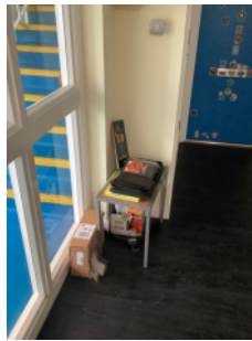
Combustible items were noted on the first floor common corridor
