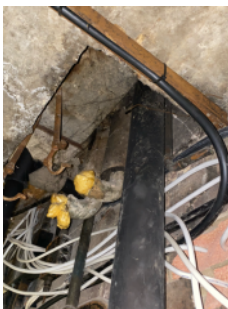
Fire stopping required in the basement
