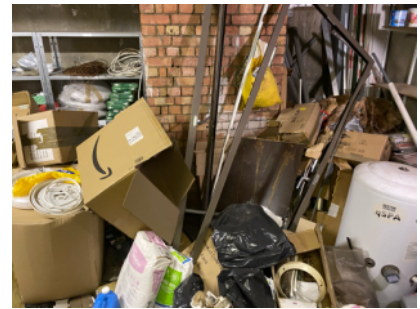
The fire-loading in the basement area is unacceptable.
