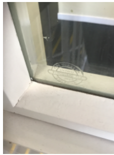
FR Glazing on staircase door glazing
