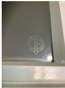
FR Glazing on staircase panels
