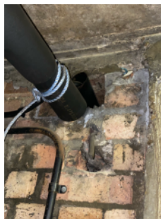
Fire stopping required in the basement
