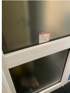
Certification of FR glazing in side panels to flat entrance doors
