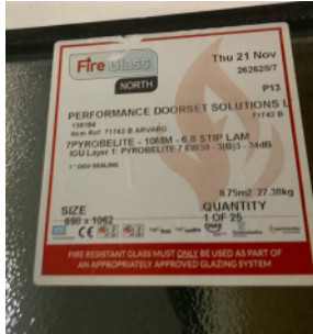
Certification of FR glazing in side panels to flat entrance doors
