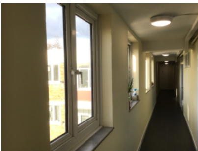
Openable windows on corridors
