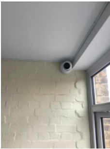
CCTV is installed on all levels
